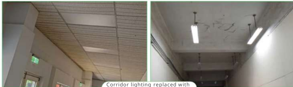
Corridor lighting replaced with 20W lights or panel lights
