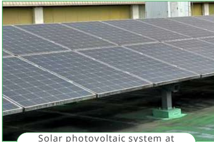
Solar photovoltaic system at Linkou Plant
