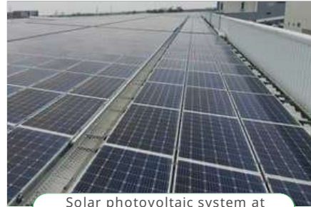
Solar photovoltaic system at Chiayi Plant
