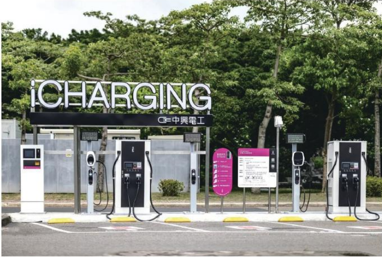
iCharging Station for Rest Stops on Highway
