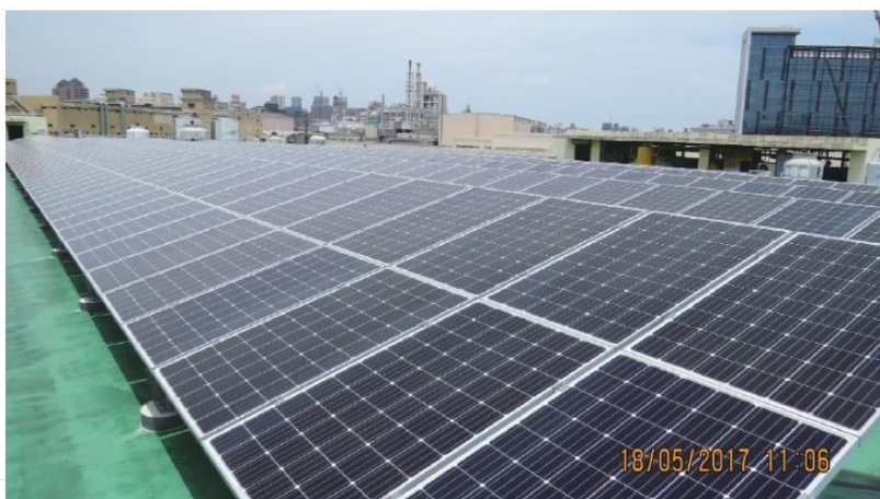
CHEM's Self-Built Solar Panel Installation for Renewable Energy in Practice
